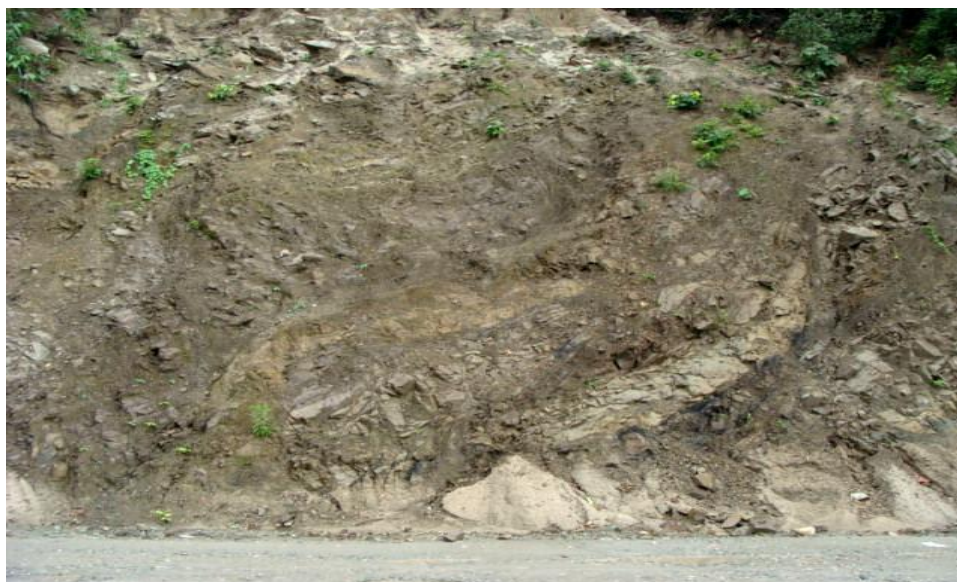
Plate 1. Upper view of Kalijhora slide, slide face are situated along NH 10.
