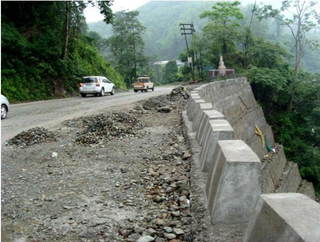
Plate 2. Road damaged due to Kalijhora slide and toe erosion of Teesta River.
